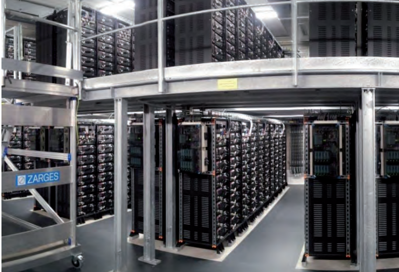
Figure 3.3.3.2.5: Interior view of the first commercial battery power station in Germany. The 5 MW lithium-ion facility has the equivalent reserve capacity potential of a conventional 50 MW turbine. | Source: WEMAG.
