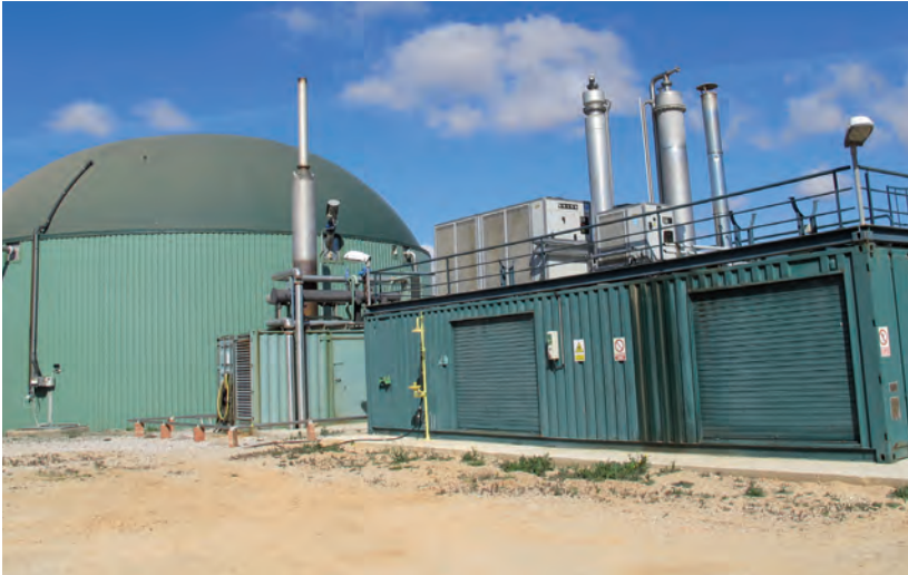
Figure 3.1.5.2: A biogas-producing anaerobic digestion plant. | Source: RENAC.
